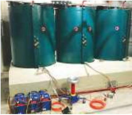
Figure 3: PD test setup using CPC 100 as HV source and the MPD 600 PD Analysis System.
