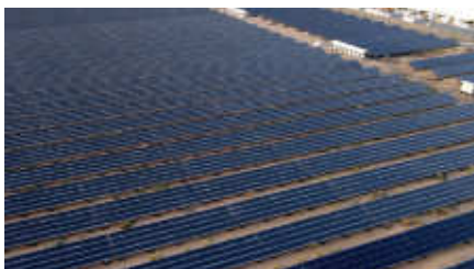
The system features nearly 23,000 Cat PVT117 photovoltaic modules
