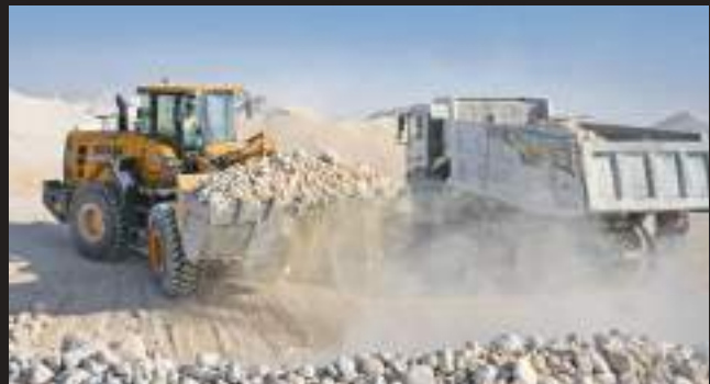
The L958F is responsible for loading the wadi stone (hard limestone pebbles that measure up to 30cm in circumference) into tipper trucks for delivery to the site's crusher hoppers.
